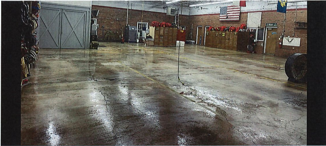
Concrete would move and shift as trucks drove in and out.
