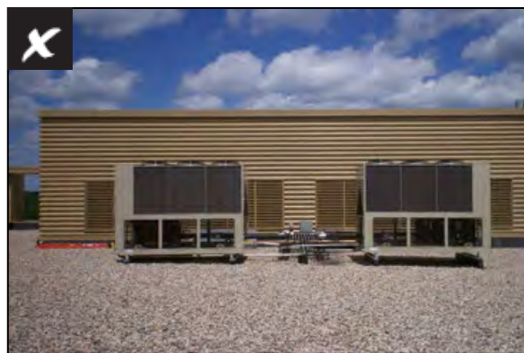
Unscreened roof-top equipment
