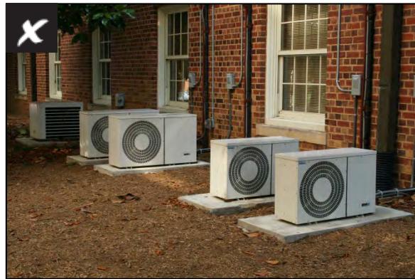
Unscreened ground-level equipment
