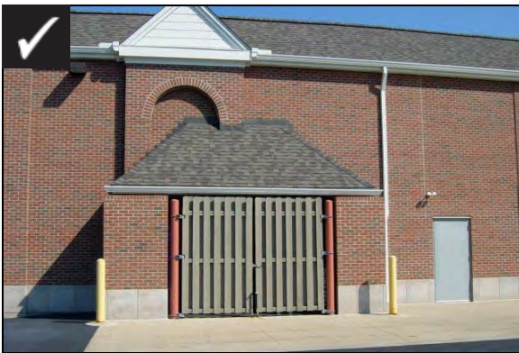
Screened ground-level equipment
