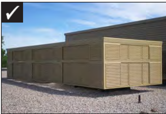
Screened roof-top equipment
